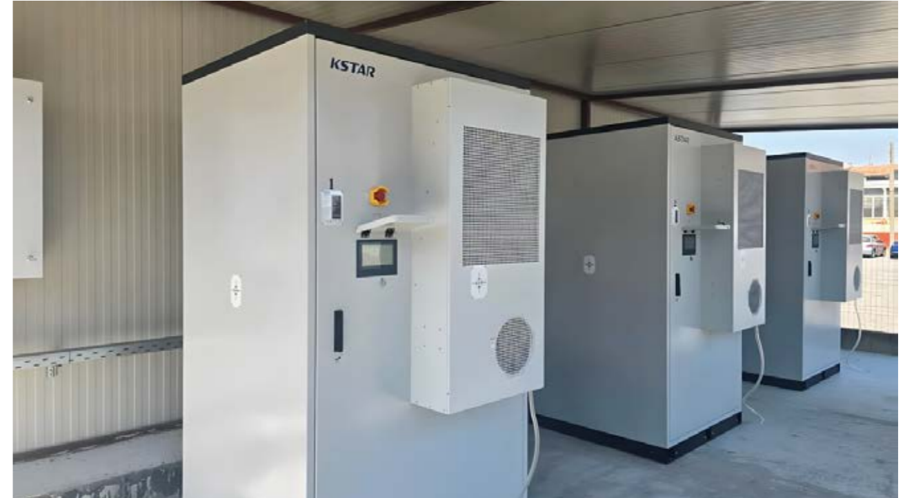
03 C&I ESS Project in Bulgaria
