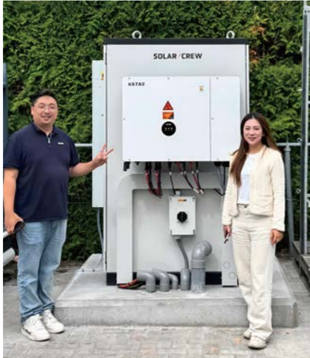
01 C&I ESS Project in the Netherlands
