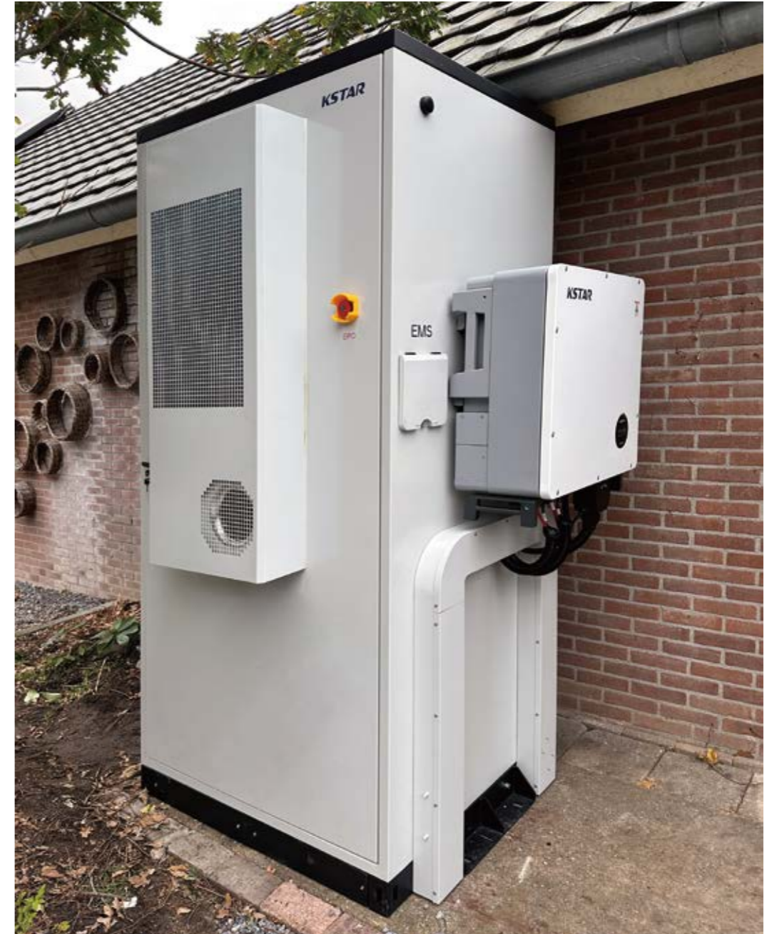
08 C&I ESS Project in the Netherlands
