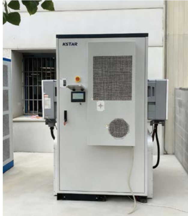
02 C&I ESS Project in Spain
