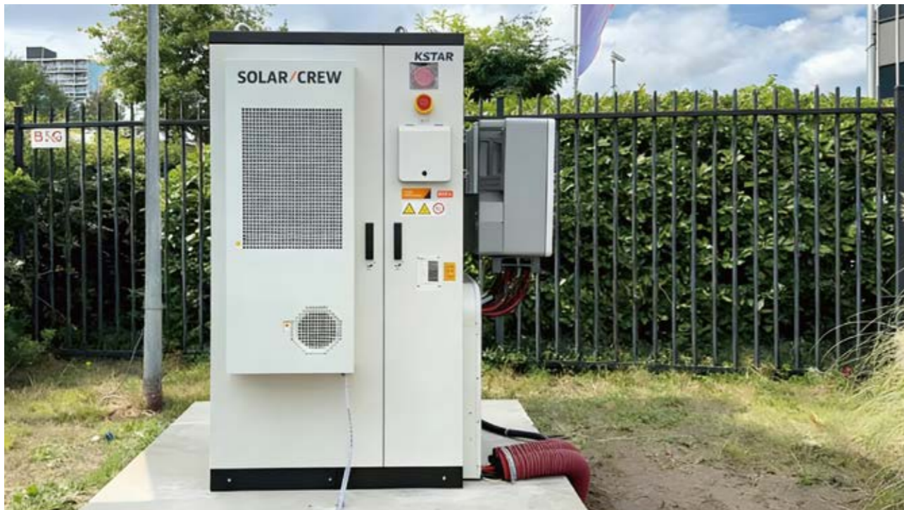
04 C&I ESS Project in the Netherlands
