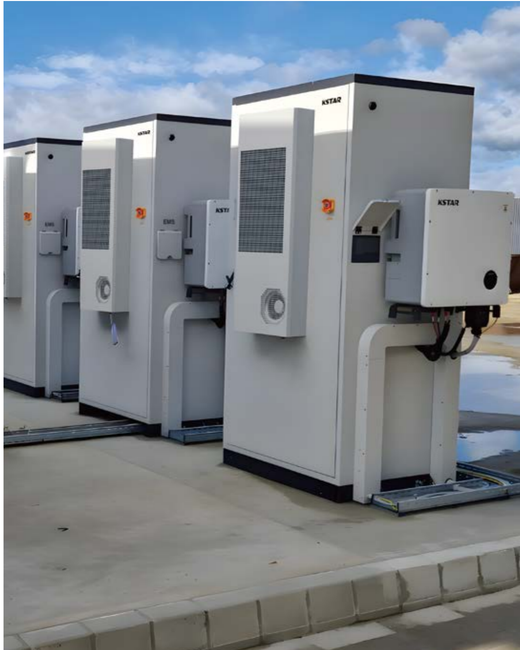
07 C&I ESS Project in Hungary
